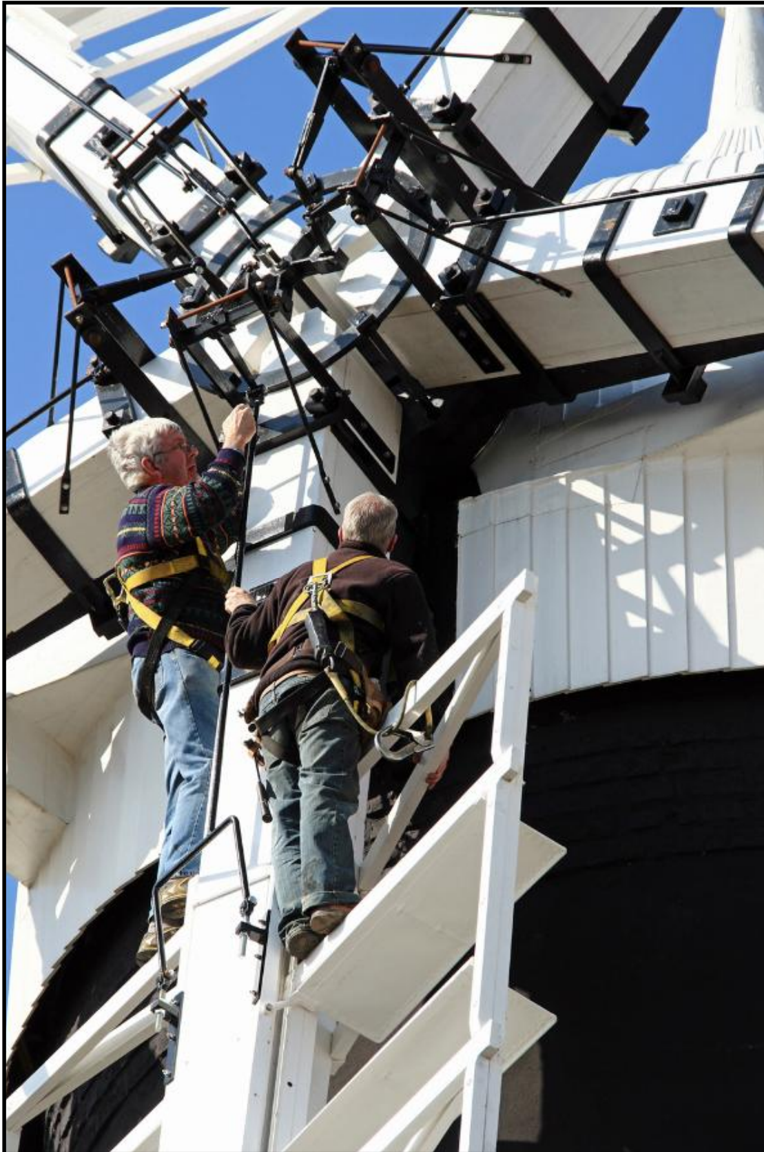
Assisted by one of the Friends of the Windmill, Tom Davies adjusts part of the front striking gear at Holgate Mill, York. The photograph shows the operating gear and fixings for five double-sided cross-mounted sails. Here, all the cast iron and steel (formerly wrought iron) components are decorated black.
