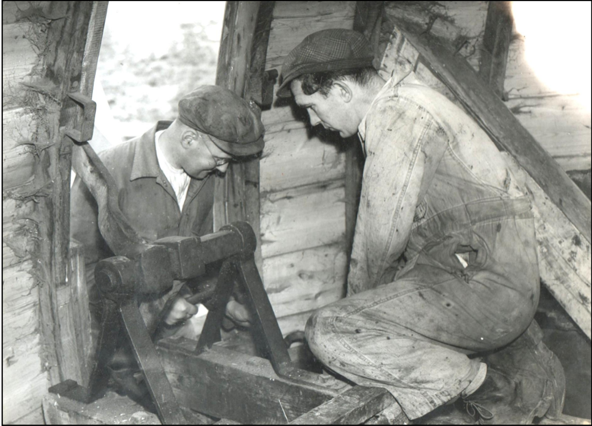
Bob Thompson and a young Jim Davies are pictured at work inside the rear of the cap of Skidby tower mill. Bob was Jack's stepbrother and may have been disappointed not to eventually inherit the business. This photograph must have been taken soon after Jim joined the business once he had been demobbed following WWII.
