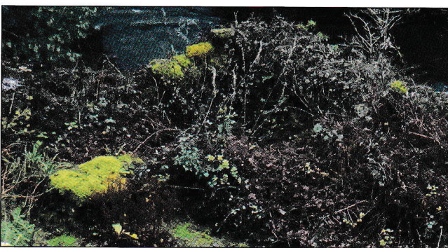
Fig. 1. In 2017 the ruins were further dilapidated and extensively overgrown.
