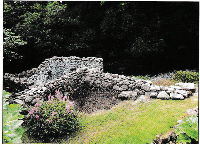
Fig. 3. By mid-2021 the mill was fully cleared, stabilised and lime mortar pointed where required.
