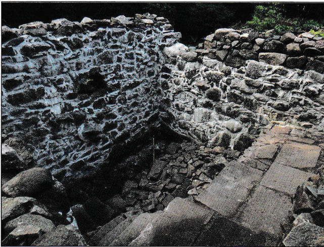
Fig. 6. View of internal head race and water channel. Yellow pole shows position of central spindle bearing.
