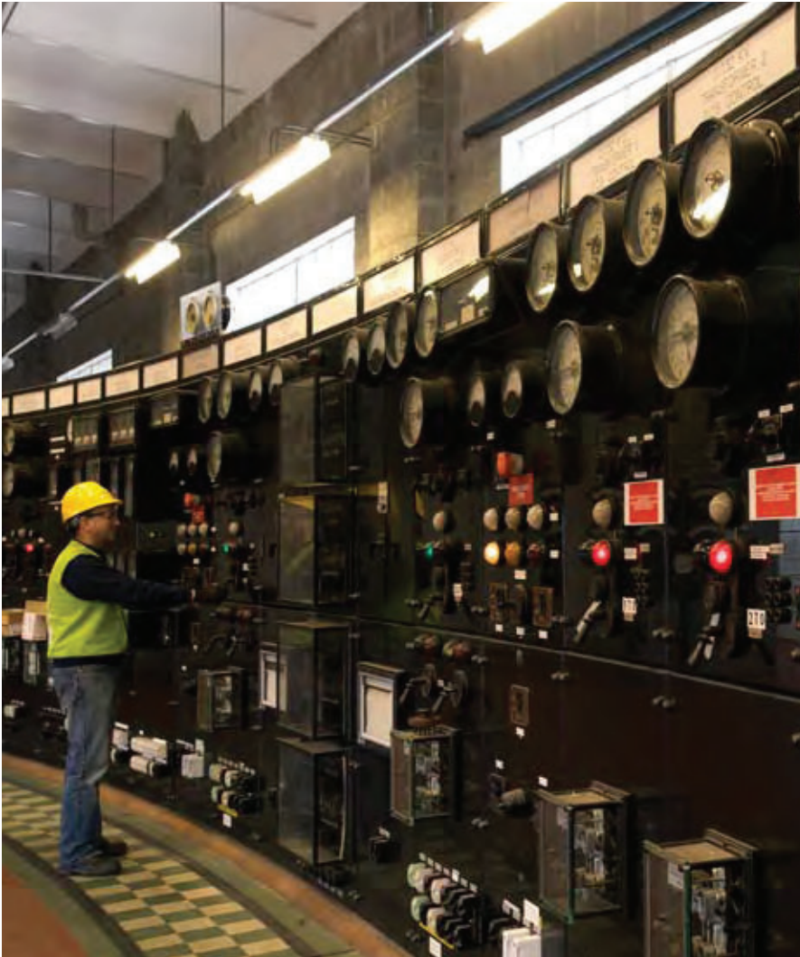
7.7 Detail of the control panel at Tummel Bridge power station, 1933, Tummel and Rannoch hydroelectric scheme.
