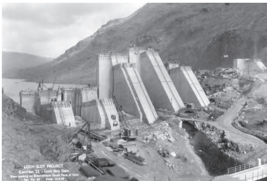
6.2 Downstream face of Sloy dam under construction, 1949, Sloy hydroelectric scheme. © Scottish and Southern Energy
