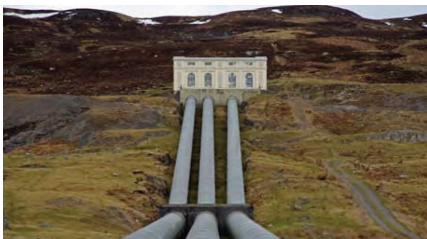
5.2 Rannoch valve house, 1931-3, Tummel and Rannoch hydroelectric scheme.
