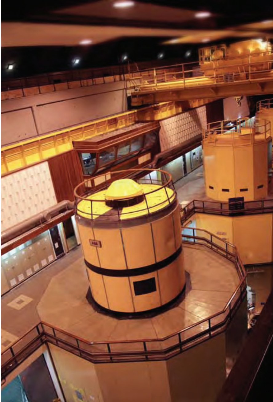
6.5 100 MW turbine, Ben Cruachan turbine hall floor, 1965, Sloy / Awe hydroelectric scheme.
