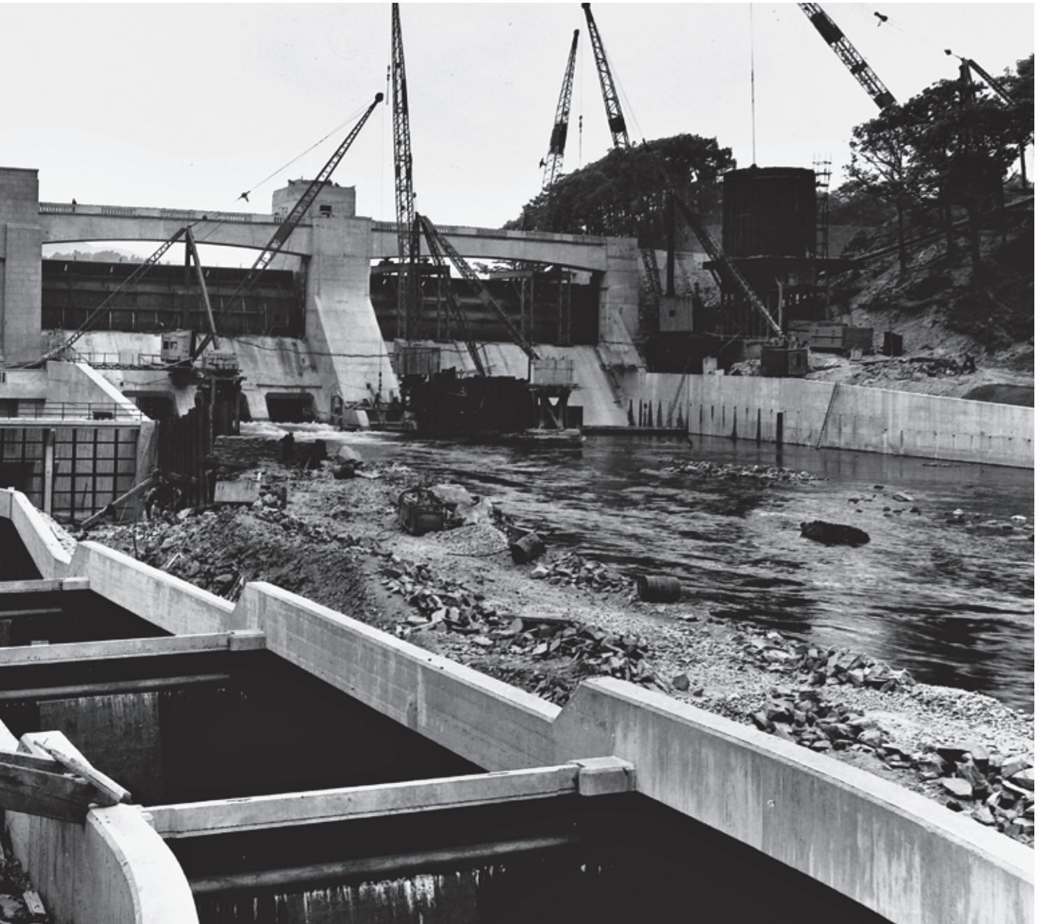
4.5 Pitlochry power station under construction, 1950, Tummel Valley hydroelectric scheme. Crown Copyright: RCAHMS. Licensor www.scran.ac.uk
