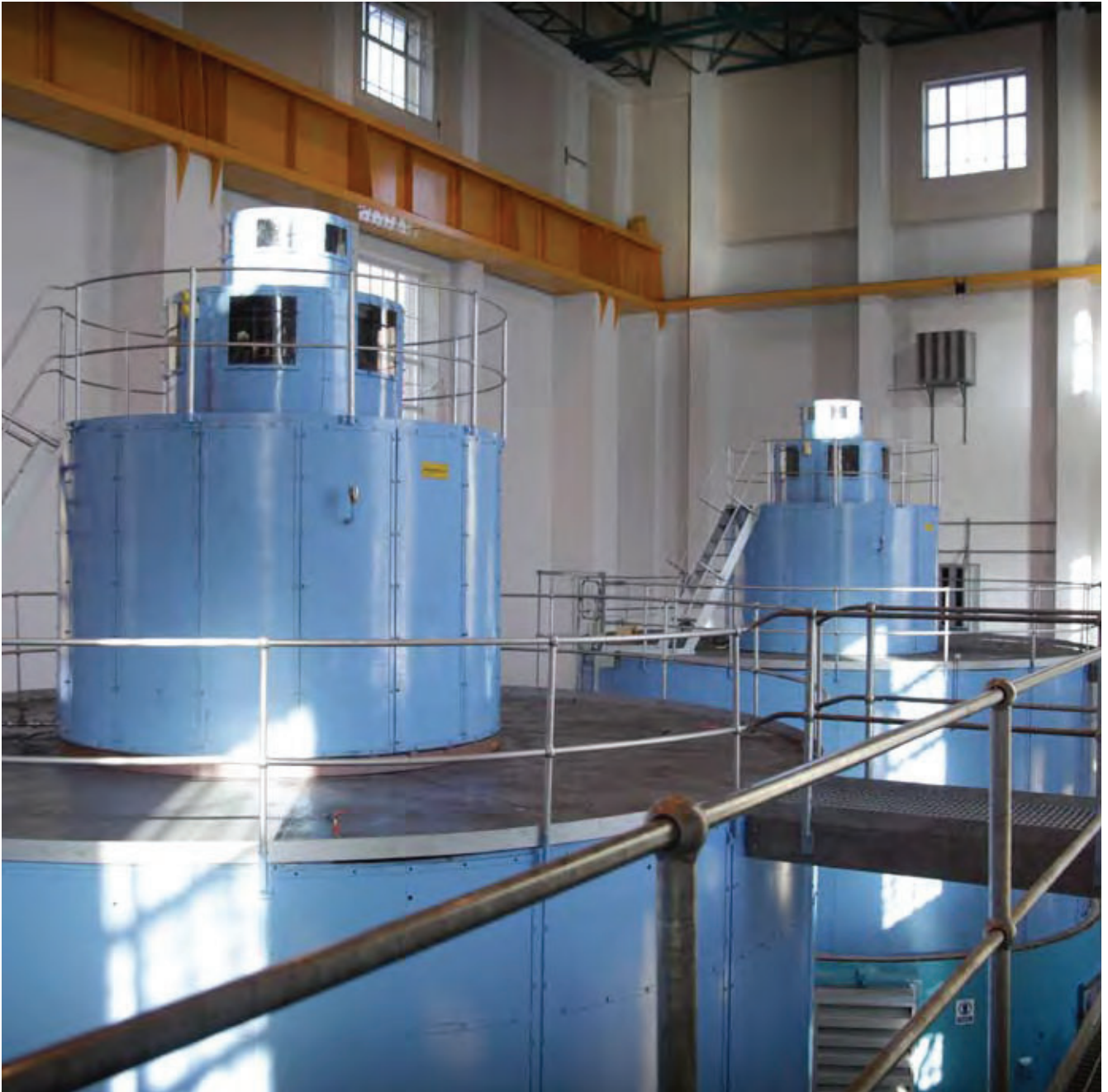
7.6 Interior view of Fasnakyle power station, 1950, Affric hydroelectric scheme.
