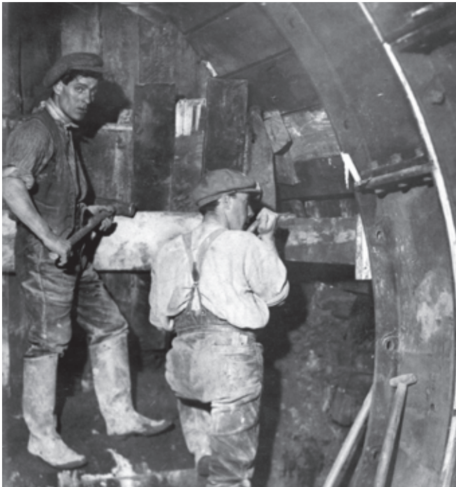
2.4 Workers constructing the tunnel at Bonnington power station, 1926, Falls of Clyde hydroelectric scheme. Crown Copyright: RCAHMS. Licensor www.scran.ac.uk
