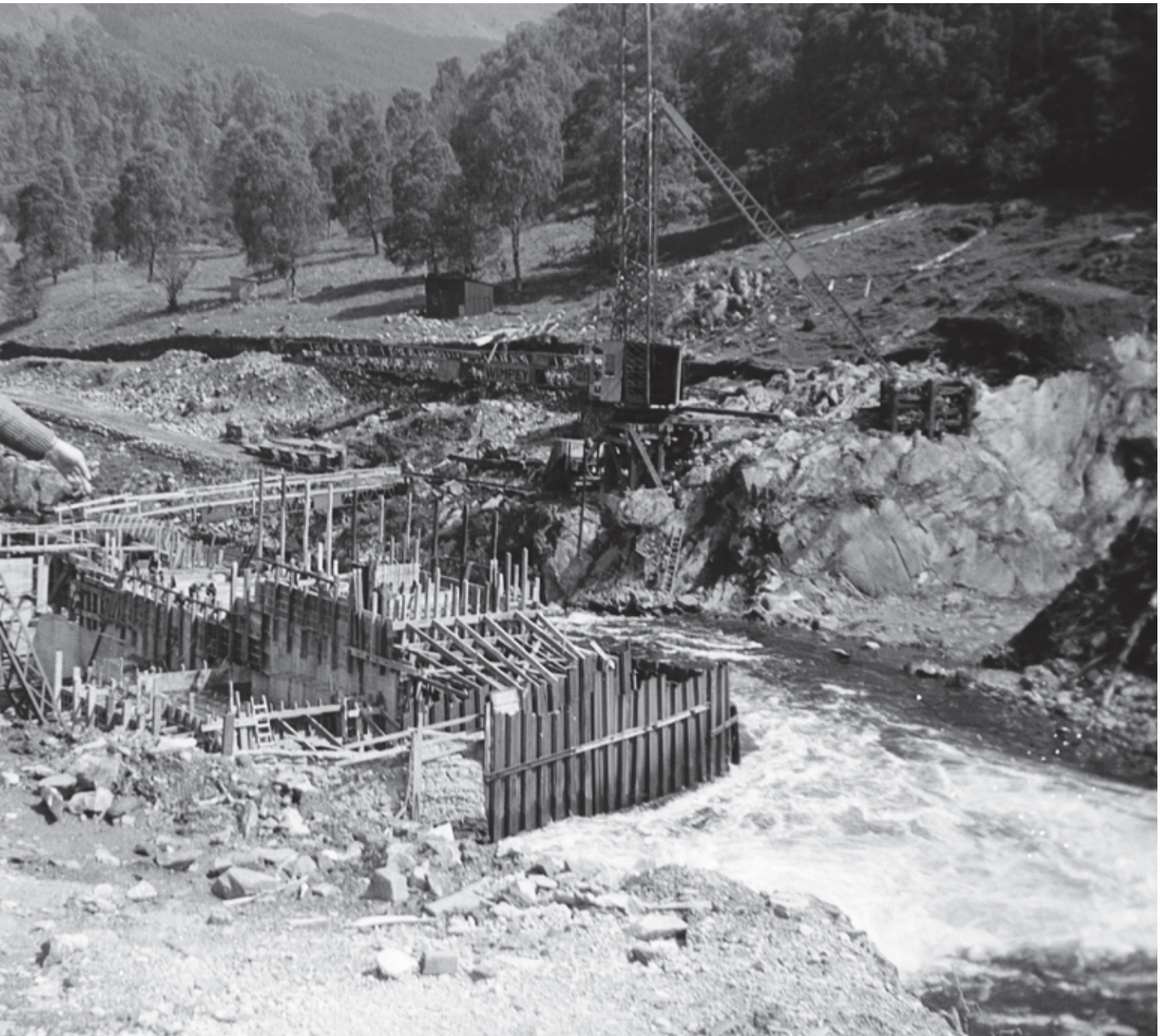
7.5 Construction work during the building of the Tummel Dam, 1947, Tummel Valley hydroelectric scheme. © National Museums Scotland
