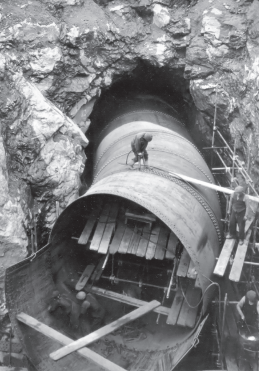
3.6 Construction work on the tunnel at Sloy, 1943-50, Sloy hydroelectric scheme. © Scottish and Southern Energy
