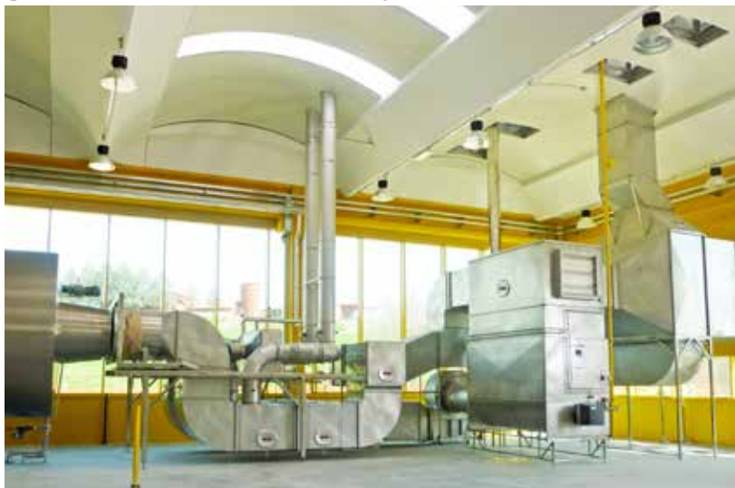
Figure 3 – Ventilation technology of a 10 ton Schulz malting system; installed at Mastri Birrai Umbri Coop. ARLI Umbria (Italy)
