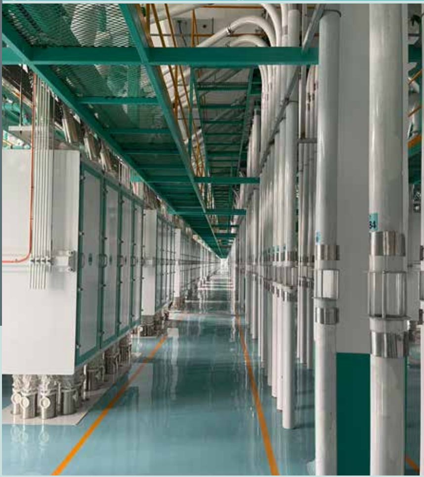
The vast range of equipment featured at the Suiping facility includes purifiers and planifiers supplied by Swiss manufacturing company Bühler
